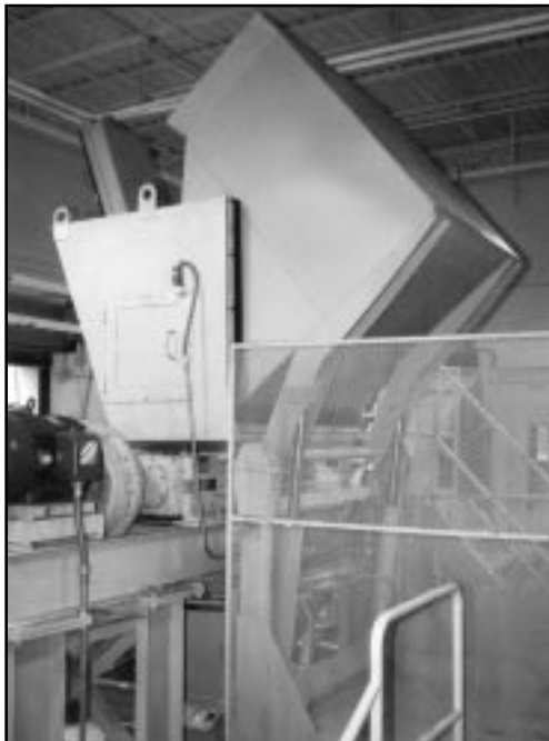
complete systems including shredders, conveyor systems, tipplers, platforms, and much more. This system is used for medical waste destruction
